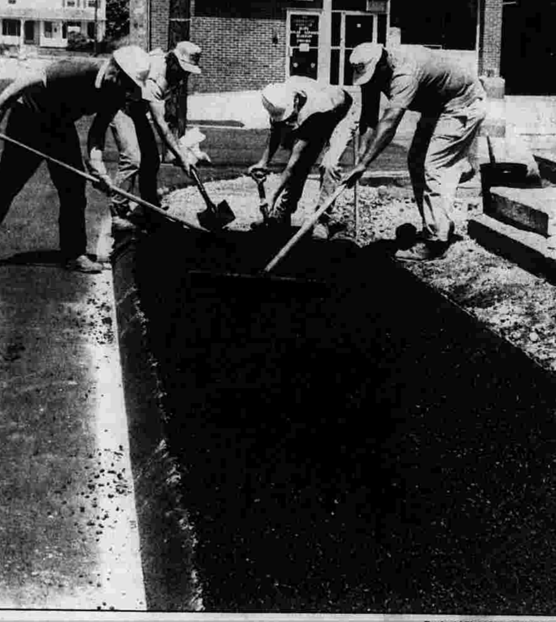
BACK WALK — Laborers from The Ball Co. even off the coat of asphalt for a sidewalk along the bypass road for the downtown Manchester reconstruction. Replacement of some utility lines will constrict or close Main Street to traffic at various times.
